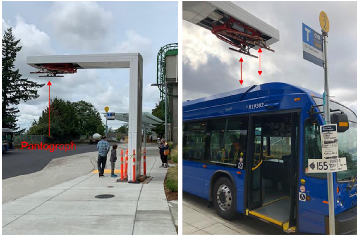
Figure B-5 Typical In-route Charger Installation
