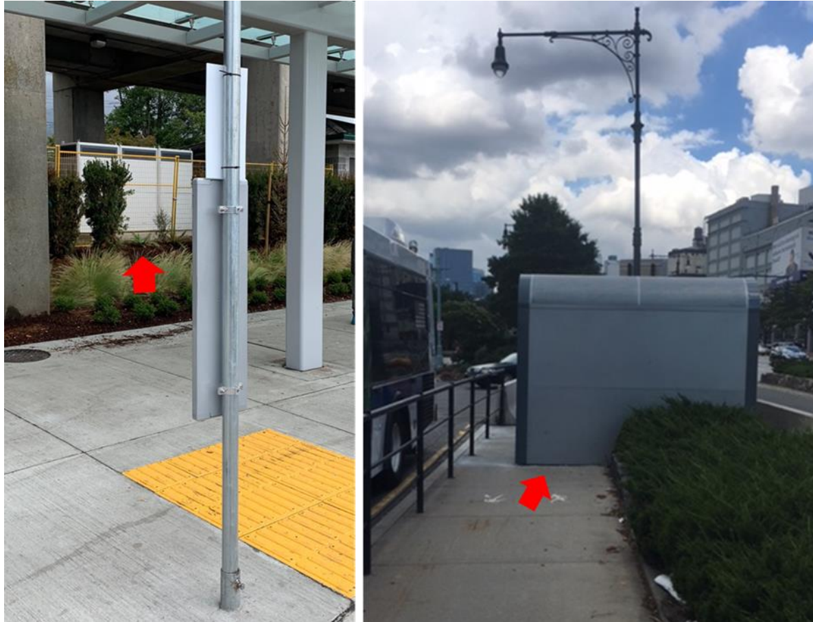
Figure B-6 450 kW In-route Charger Power Modules
