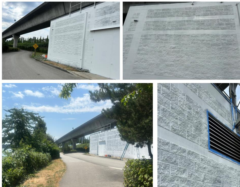
Figure 2: After nano paint application
