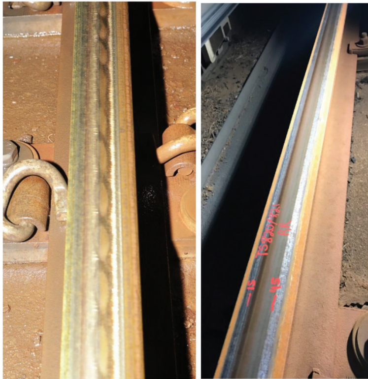
Figure 3 Corrugated rail (left) vs normal uncorrugated rail condition (right)
