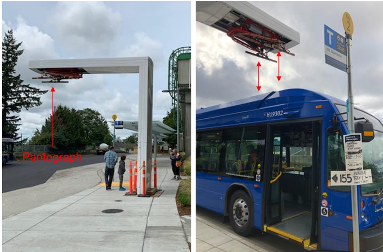
Figure B-5 Typical In-route Charger Installation
